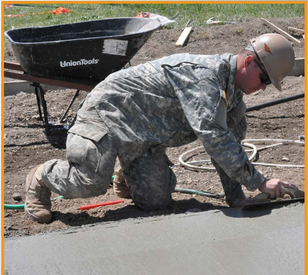
Pfc. Parker Herring places fine touches on a concrete pad that Soldiers of the 835th Engineer Detachment and 897th Engineer Detachment poured during annual training.
