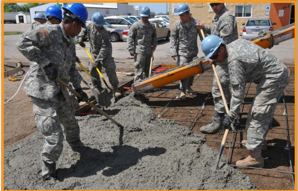
Soldiers of the North Dakota National Guard’s 835th Engineer Detachment (Asphalt Team) and 897th Engineer Detachment (Concrete Section) place concrete during annual training June 8 in Steele, North Dakota.
