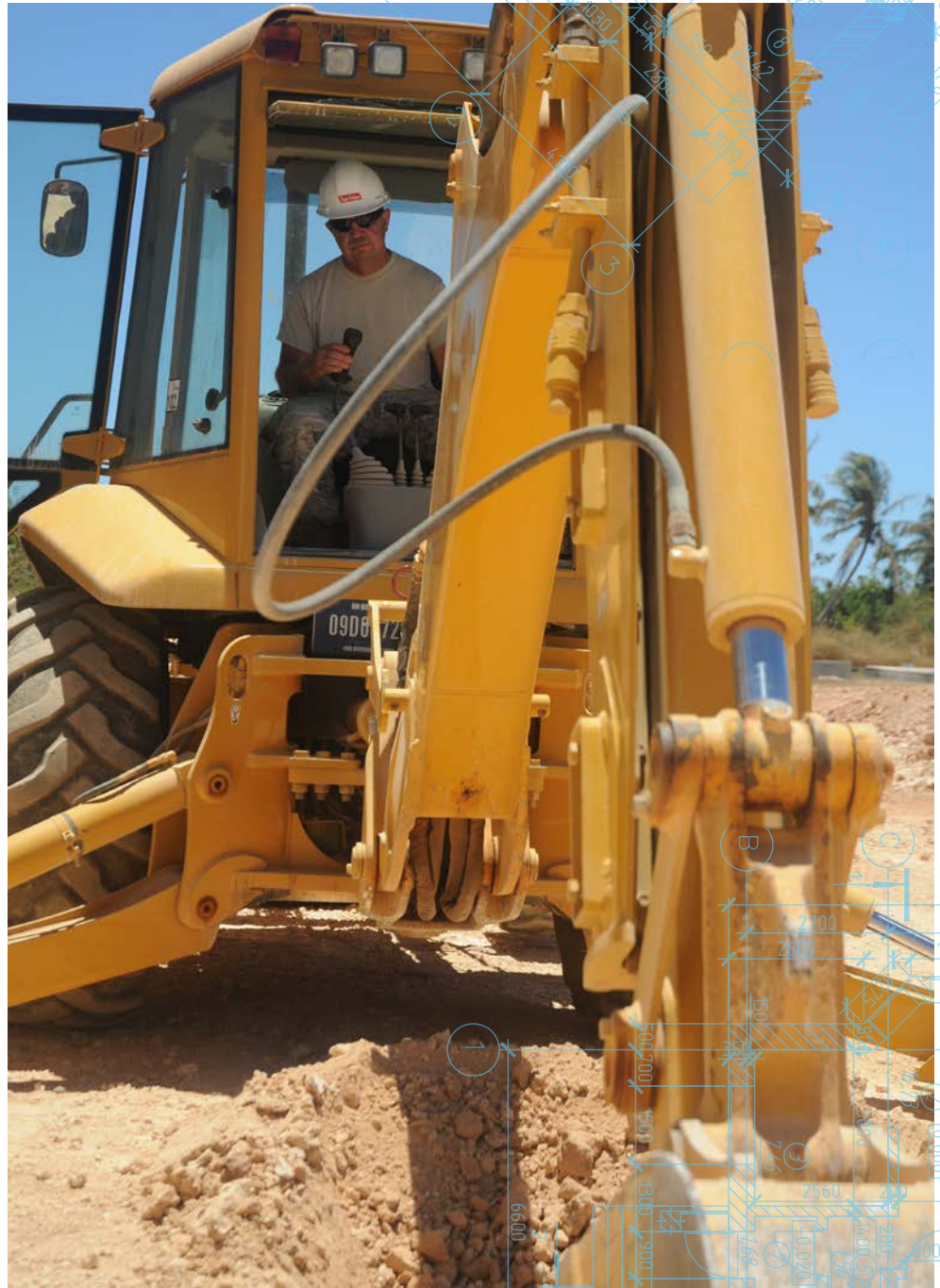
Chief Master Sgt. Scott Wagner, of the 119th Civil Engineer Squadron, operates a backhoe during an Air National Guard Deployment for Training event in Guam.
