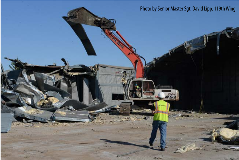
The 119th Maintenance Squadron engine test facility, better known as the hush house, at the N.D. Air National Guard Base in Fargo, is partially demolished May 17 by a contracted civilian crew.
