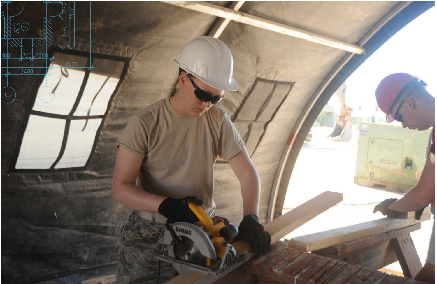
Staff Sgt. Sophie Miller, of the 119th Civil Engineer Squadron, cuts boards with a power saw May 24 on the Northwest Field portion of Anderson Air Force Base in Guam.
