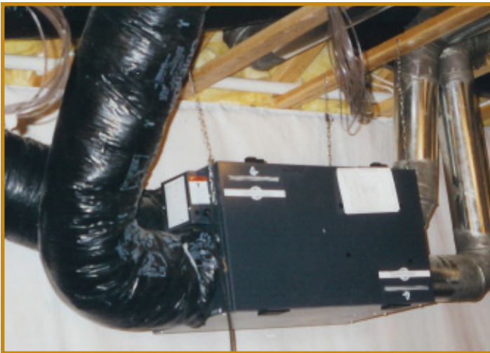
Figure 13-A. Typical installation of a heat exchanger. (Photo courtesy of Shirley Neimayer, University of Nebraska - Lincoln).
