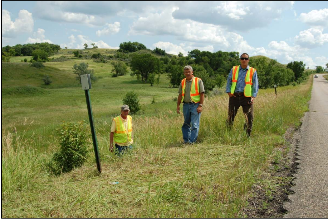
Figure 5.18 Roadway in-slope slough
