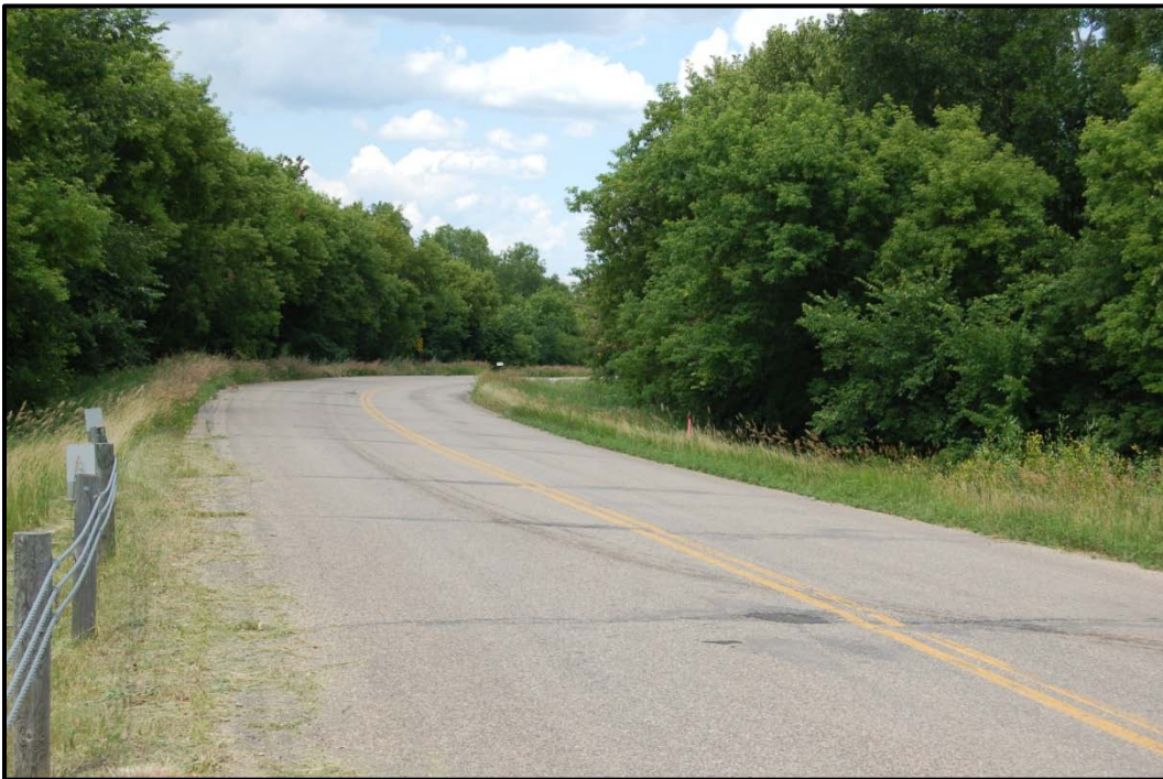
Figure 5.16 Clear zone encroachment due to vegetation
