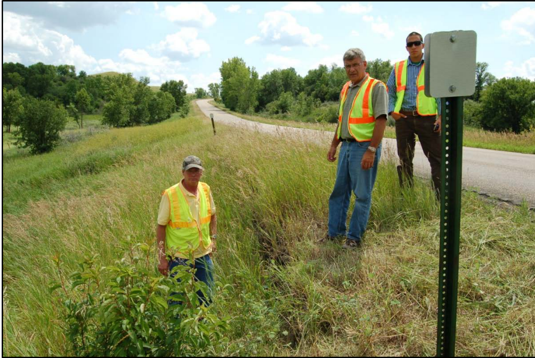
Figure 5.17 Roadway in-slope slough
