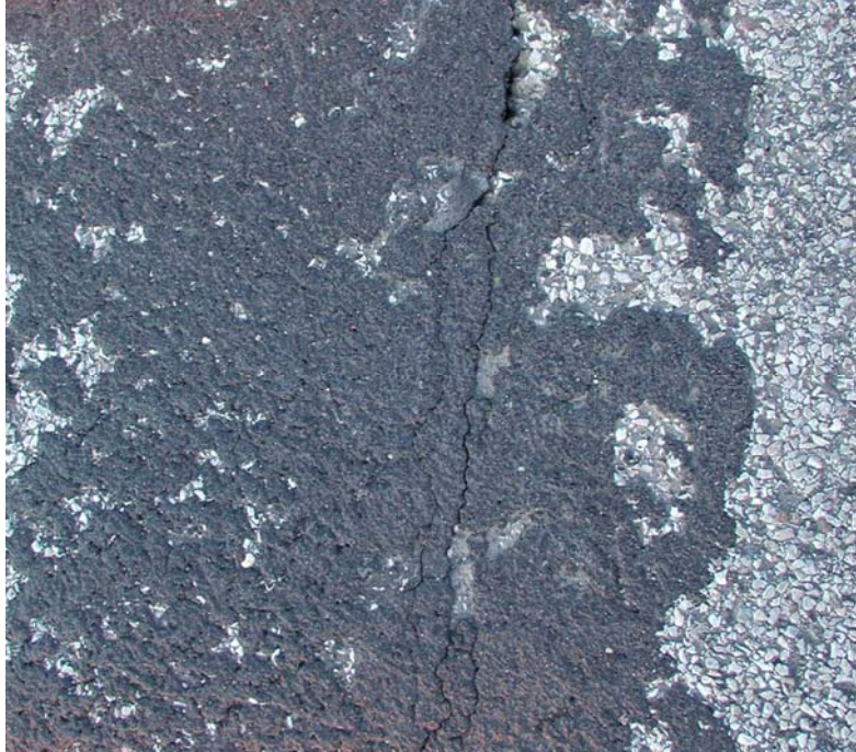
Figure 4.8 US-26 (MP 1.585) Adhesion Failure with Pullouts
