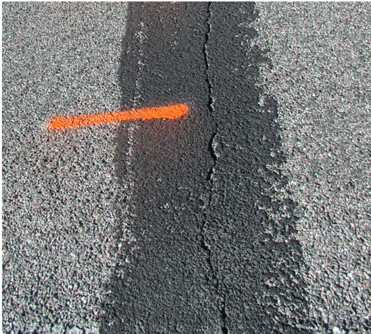
Figure 4.10 I-25 (MP 72.862) Adhesion Failure Throughout Traveled Way
