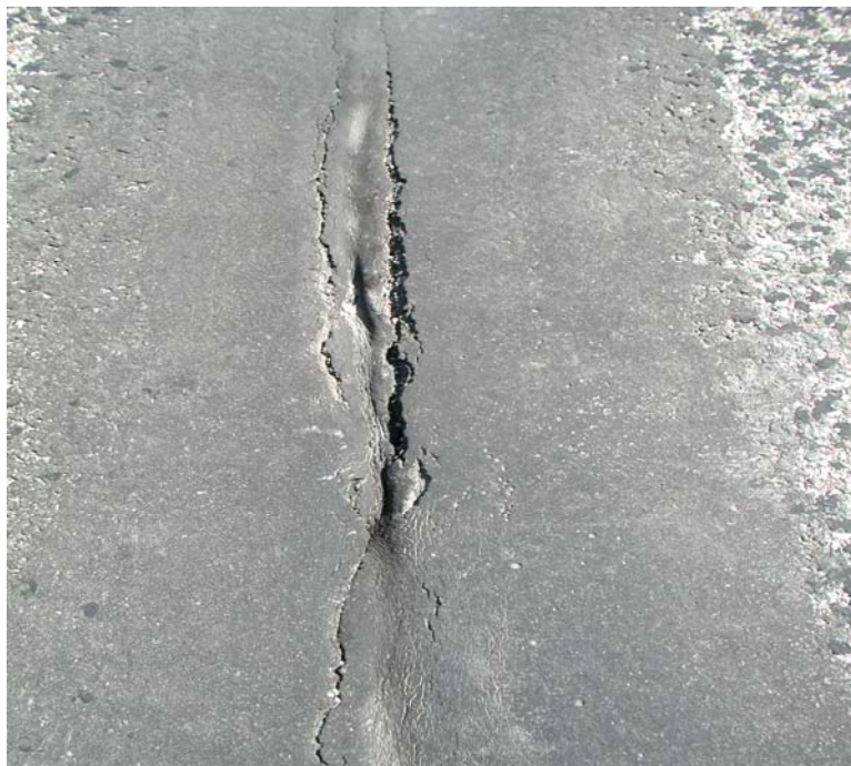
Figure 4.4 WY-93 (MP 19.611) Adhesion and Cohesion Failure
