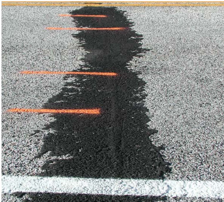
Figure 4.7 US-26 (MP 5.700) Edge Deterioration Throughout Traveled Way
